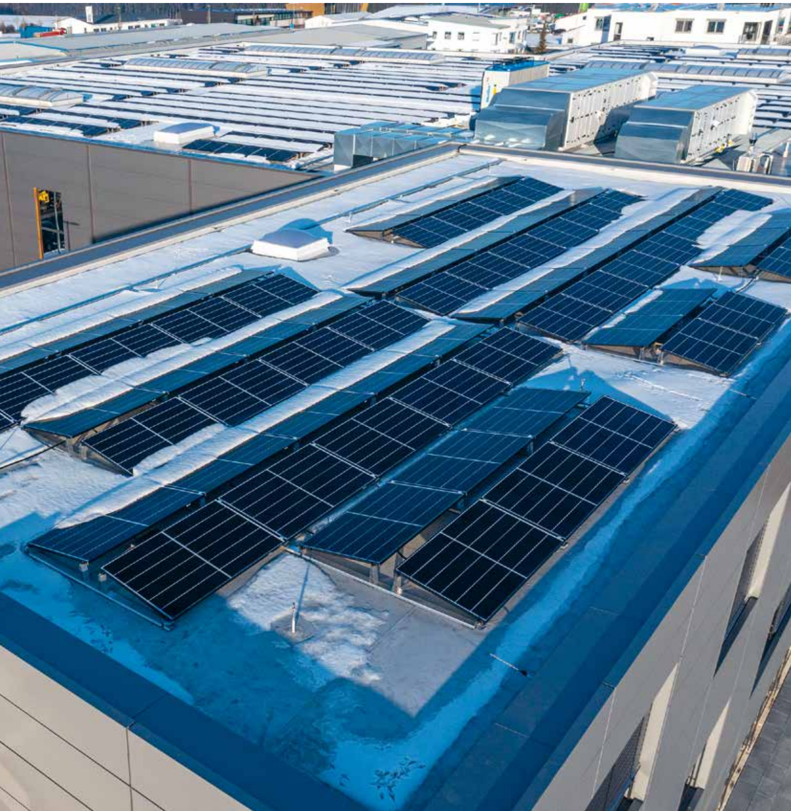
PHOTOVOLTAIC SYSTEM ON THE ROOF OF ZEISER GMBH IN EMMINGEN When new investments are made, sustainability aspects are given substantial weight alongside purely economic considerations.
